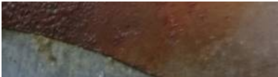
Fig. 2. Element of the mobile platform with various levels of corrosion intensity
