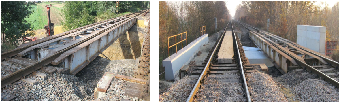
Fig. 1. View of the track on the bridge, visible two relieving constructions built in both tracks
