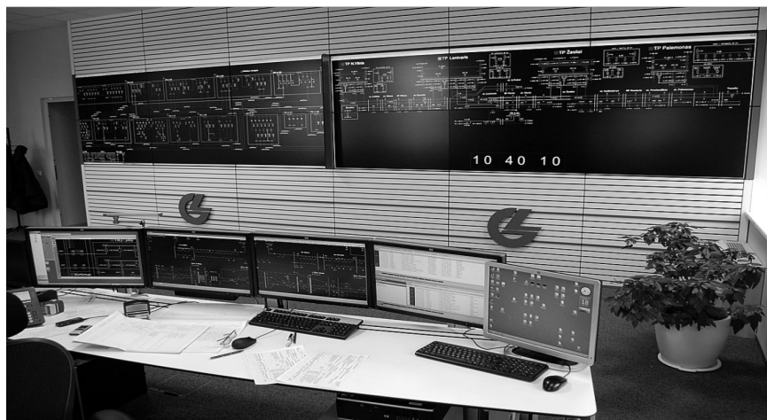
Fig. 10. A photo of LG contact network equipment remote control
