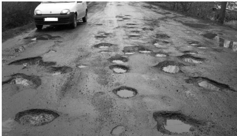
Fig. 2. Huge holes in the road Rys. 2. Wielkie wyrwy w jezdni
