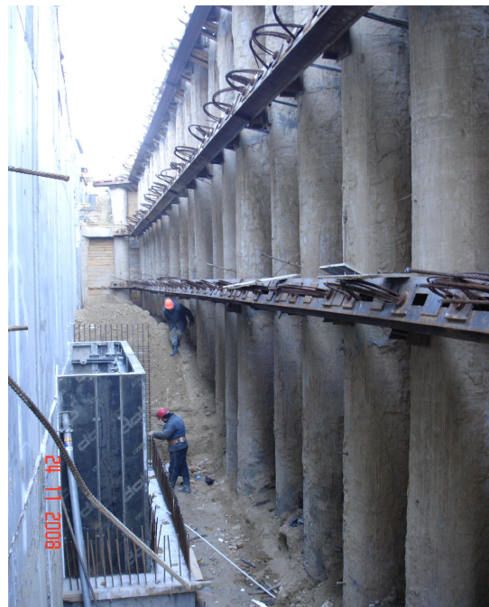
Fig. 4. Fencing of pit walls during construction of the retail and business center “Kaskad Plaza”
