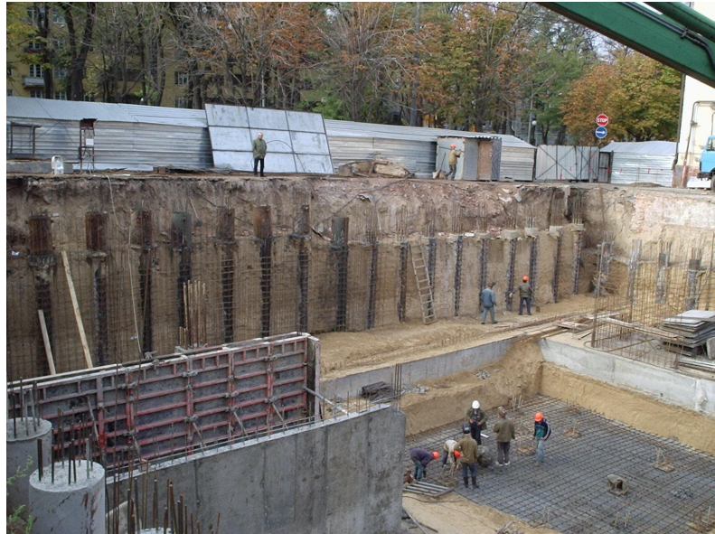
Fig. 3. Erection of underground stories of the retail and business center “Atrium” under the protection of a vertical pit fence constructed by bored reinforced concrete piles
