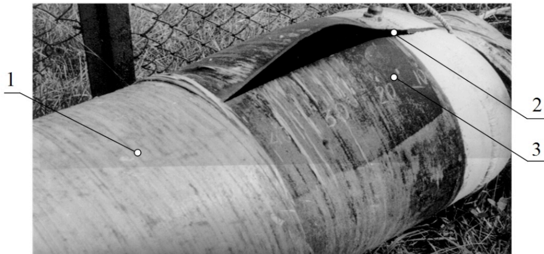
Fig. 6. Fracture pattern of a metal-fiberglass pipe: 1 – fiberglass plastic; 2 – crack; 3 – metal
